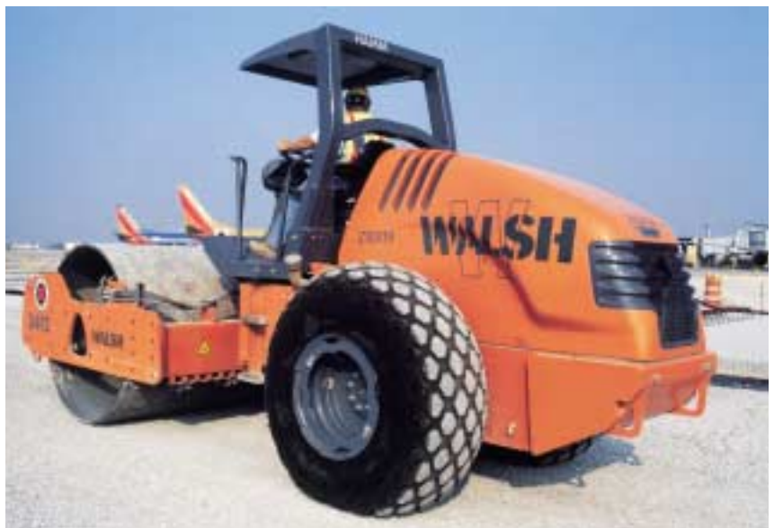
Kevin Doogan, operator for Local 150, compacts stone base on Chicago Midway Airport airfield
