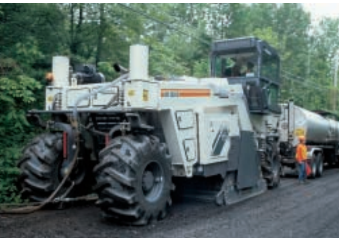
Ulster County foam-recycles over 20 miles of pavement each year; liquid asphalt is provided by tanker at right and water from tanker off margin at left
