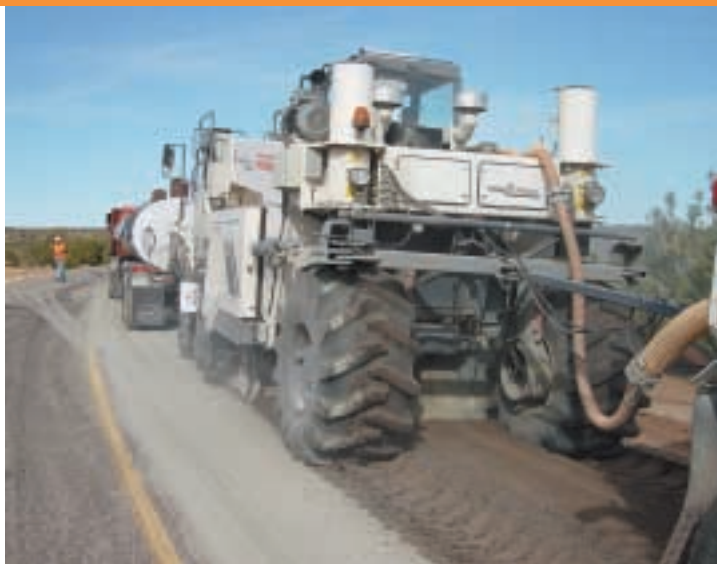
Heart of the in-place cold recycling train, the Wirtgen WR 2500 (center) pushes liquid asphalt tanker (left) while pulling water tanker (right) while in-place cold recycling pavement using 1 percent dry portland cement and 3.0 percent foamed asphalt
