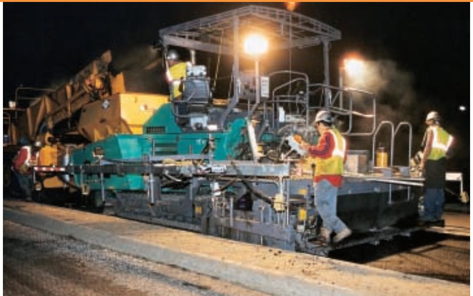
Virginia DOT requires night work for many interstate and primary route projects, Sunday through Thursday
