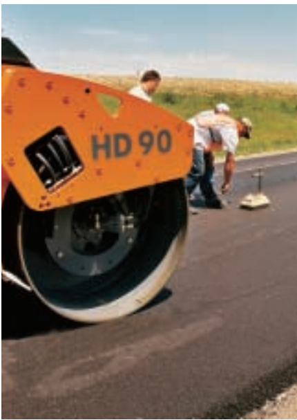
Density gauge indicated non-aggressive Oscillation compaction was achieving better compaction numbers, faster, than existing pneumatic and finish rollers combined
