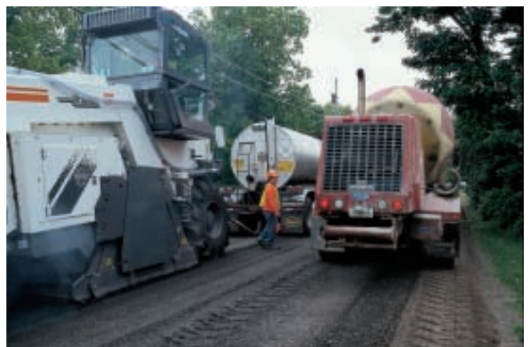
Compacted foamed base can support loads as heavy as concrete mixers immediately, while road stays open to traffic
