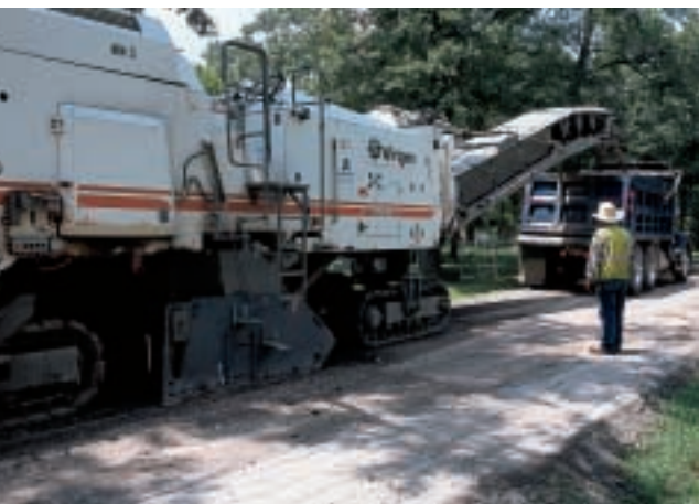
Older 2100 DC mills deteriorated pavement in unincorporated Harris County
