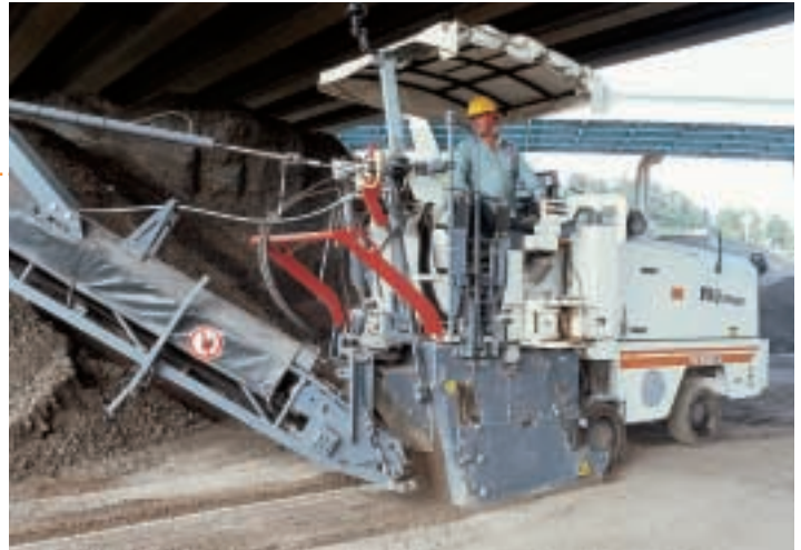
Here, St. Pete's mill removes compacted RAP from city-owned stockpile area under overpass
