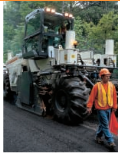
WR 2500 S can pulverize and foam reclaimed pavement in one pass, although Ulster County prefers to pulverize first, then foam
