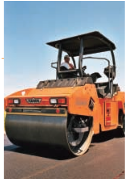
Hamm HD O90V compacts Superpave mix on ramp to Kansas 96 north of Wichita
