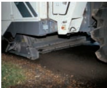
On Blue Mountain Road, liquid asphalt is added as foam at a rate of 2.5 percent per volume of reclaimed material
