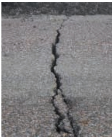
Existing deep crack is repaired by in-place stabilization, all the way to road foundation
