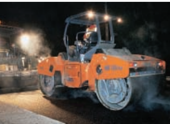
Twin high-vibration compactors bring mix to over 95 percent compaction in one or two passes, with additional passes in static mode if needed
