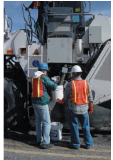
Expansion ratio and half-life of asphalt foam is checked prior to start of in-place cold recycling at Canyon de Chelly National Monument
