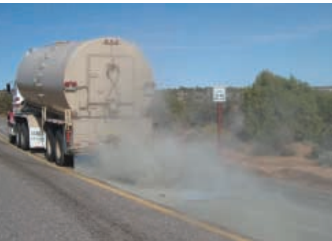
Dry portland cement is added to pavement in advance of in-place cold recycling using foamed asphalt at Canyon de Chelly National Monument
