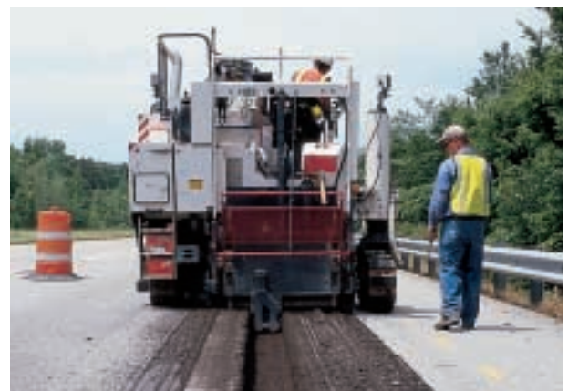
W 1200 F of Charbon Contracting uses 12-in FCS drum to cut edge drain trench
