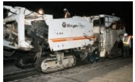
Existing pavement is milled 1.5 in deep by Wirtgen 2100 DC owned by sub Slurry Pavers, Inc., prior to SMA placement
